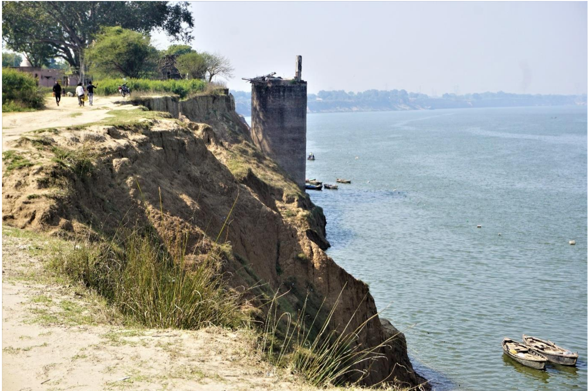
Image 62 : Eroded Ganga River Bank In Mahewa Village [Right Bank]
